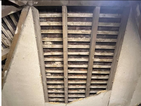
Photograph 3: partially exposed purlins, joists and slates.
